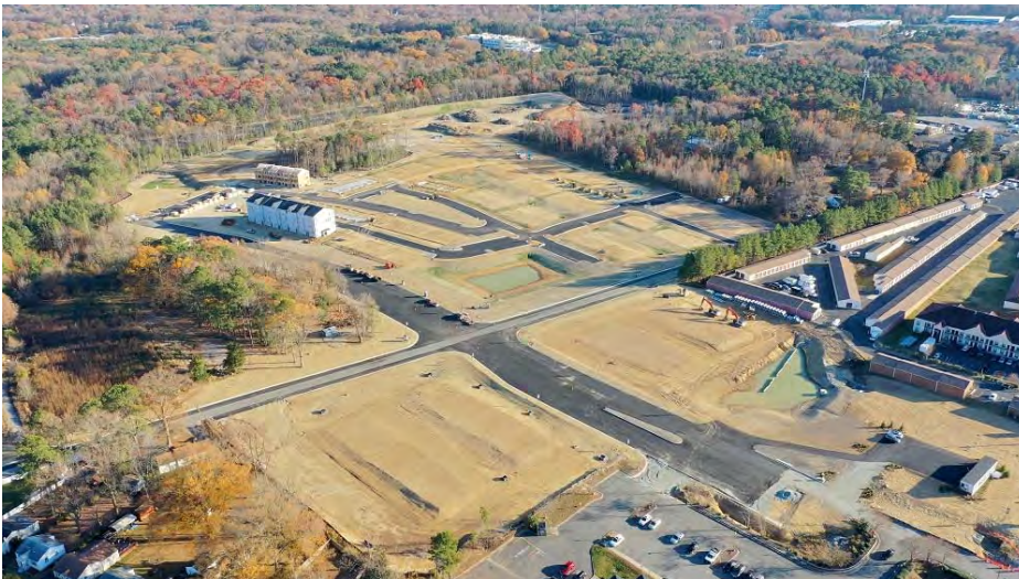
Site work for ReTreat at One has cleared land along Telegraph Road and beside I-95. ( BizSense file )
