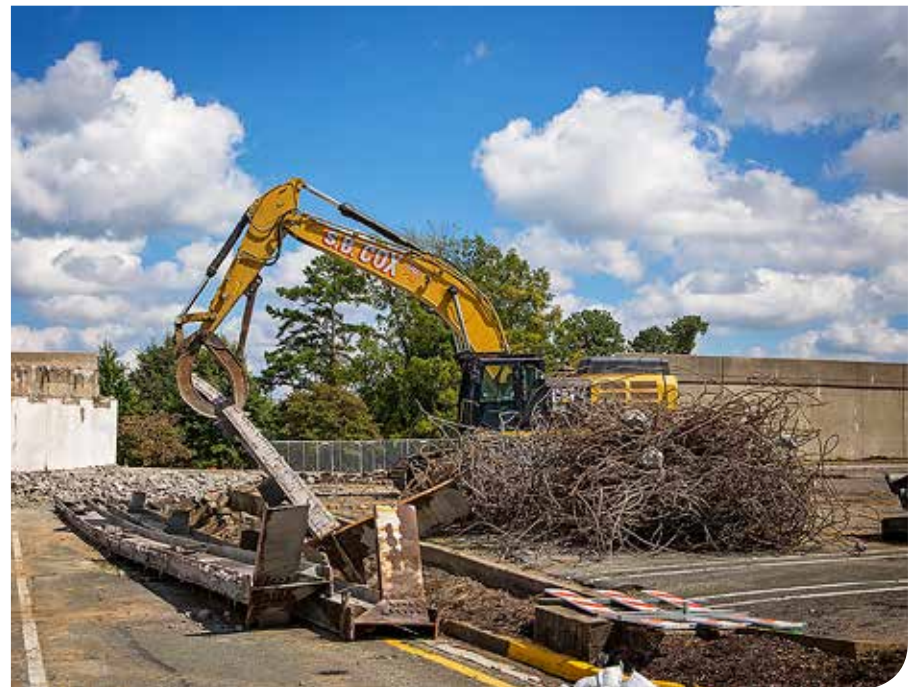
An excavator clears debris at Regency Square, following the demolition of a bridge that carried traffic from Quioccasin Road onto the mall property. A $45 million redevelopment of the mall will provide a new main entrance from Quioccasin.
