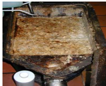
Unmaintained grease interceptor
