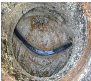
Grease buildup in sanitary sewer
