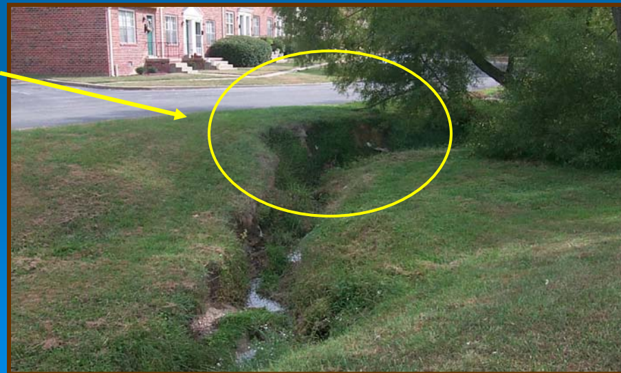
Erosion threatening parking lot integrity
