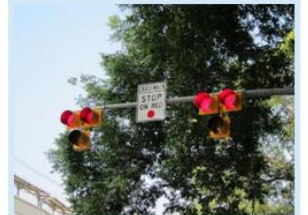
Example of PHBs mounted on a mast arm. Source: FHWA
