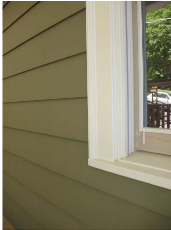
Smooth siding and traditional trim details are an appropriate choice in many of Henrico's mid-century neighborhoods.
