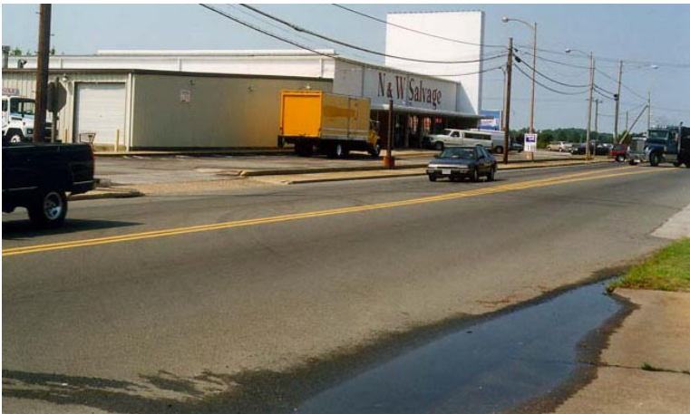
Ponding at intersections
