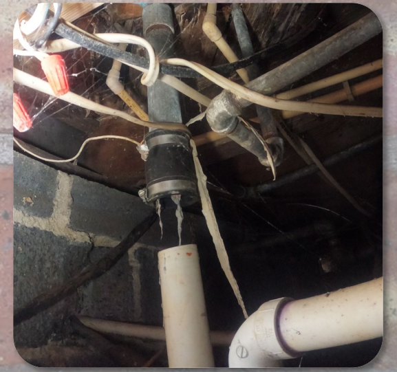
Broken Sewage Pipe
