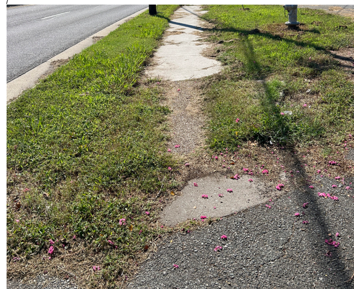
Overgrown sidewalks, not suitable for strollers or wheelchairs.
